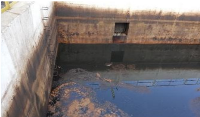
Oil layer appeared at the first flush pit.
