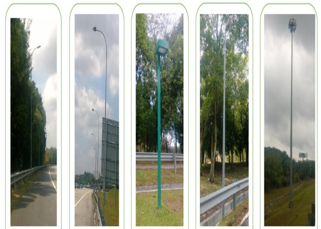
Five types of street lightings (from left to right) : LED street lighting pole, street lighting pole, compound lighting pole (type A and type B) and highmast pole.
